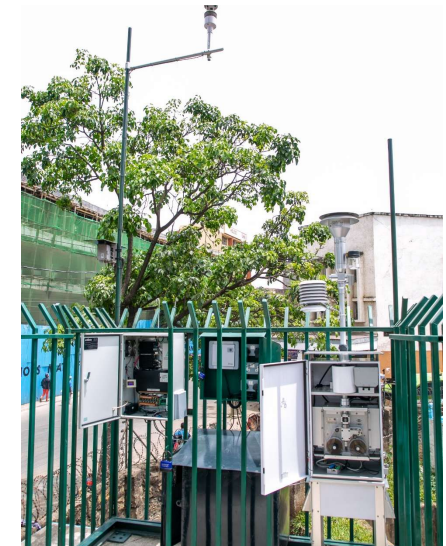
Reference Grade station set up at Fire station - Tom Mboya Street
