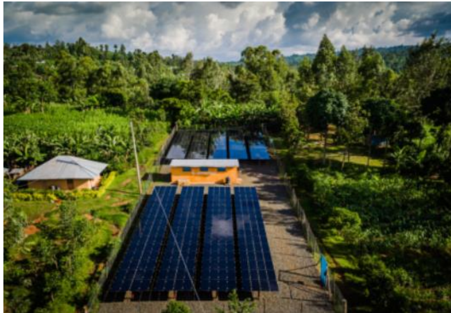
Rural solar PV minigrid
